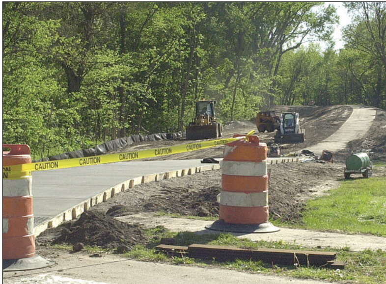
Workers take advantage of the mild spring weather by heading into the final phases of the Hebron walking trail. This 600-foot section meanders along the Little Blue River from the Fourth St. bridge west. The trail begins at Riverside Park (CCCamp) near the Hebron Sports Complex.
