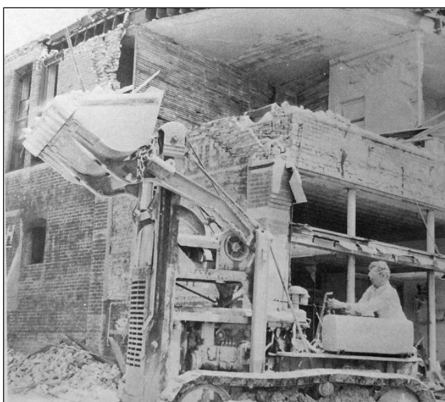
Monday, May 11 - The dozers began the task of moving the debris from the various buildings and walks into the streets where it was then loaded into dump trucks. ~The Hebron Disaster~
